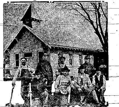
St. John's Evangelical Lutheran Church, Mexico, Mo., has but eight adult men members. They decided the church needed a new building. So they built it. Top: The building below, the men who built it.
